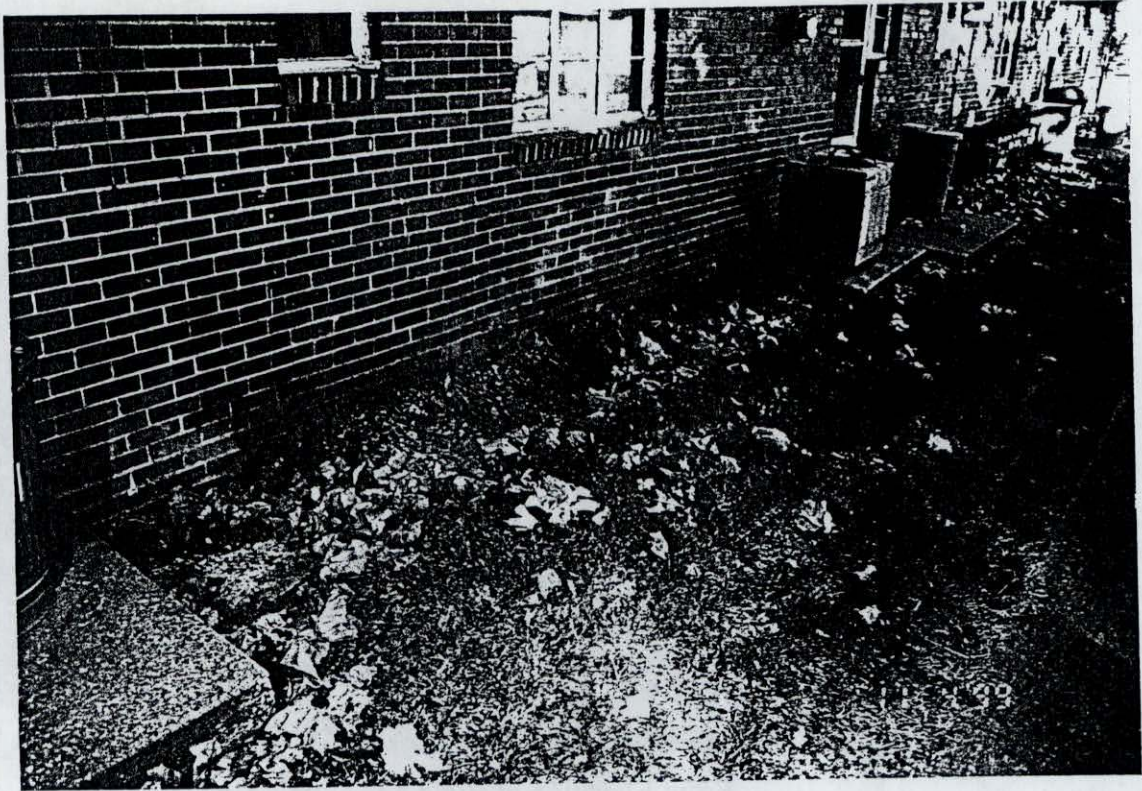
Rear Elevation of Building on 25th Avenue (Note Erosion From Lack of Gutters)
